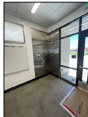
Completed Eye Wash Station
