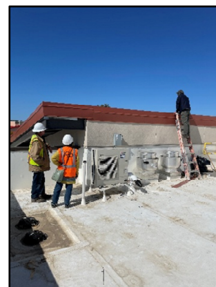
Electrical Punch Walk
