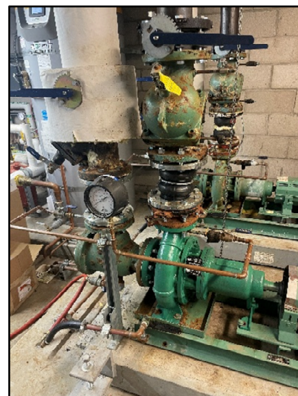
New Pump Installed
