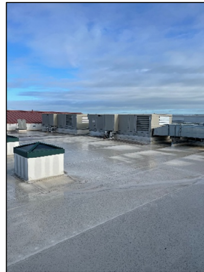
N3200 Rooftop Units
