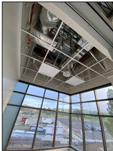
Acoustical Ceiling Grid
