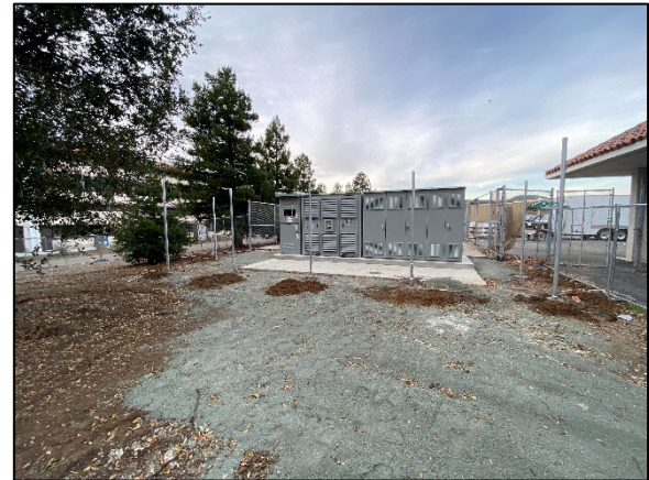
Electrical Items Installed
