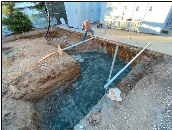
Equipment Pad Base
