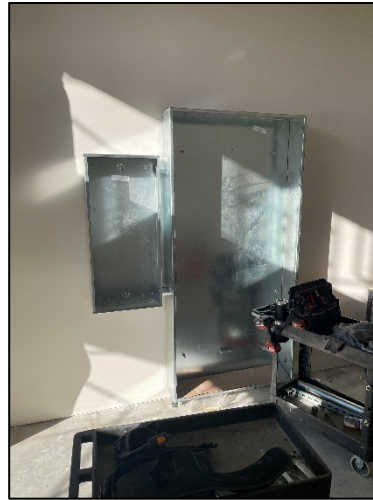
Electrical Room Panel
