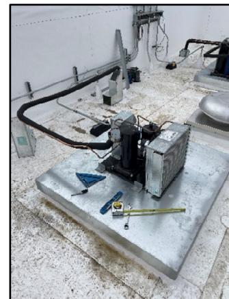
Refrigerator Freezer Lines
