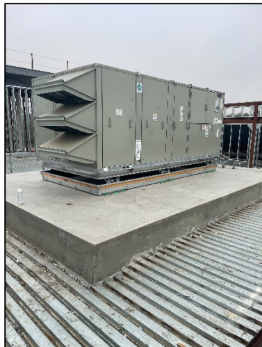
Rooftop HVAC Equipment
