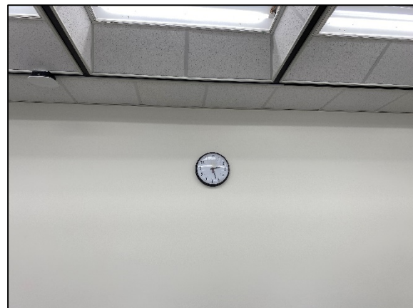
4100: Hardwired Clocks Reinstalled
