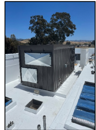
New MZU in place
