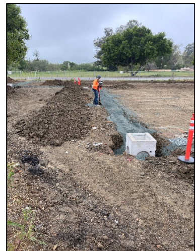
[ Parking Lot 4 Storm Drain ]
