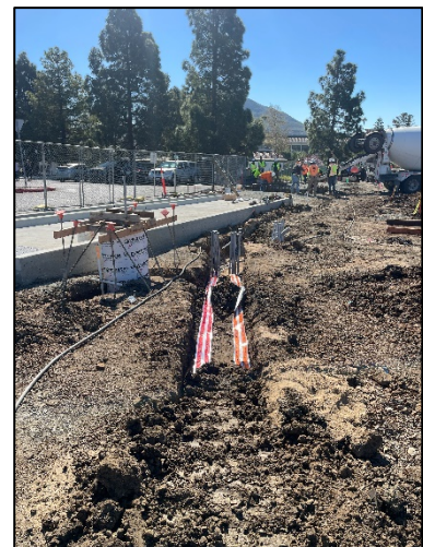
[ U/G Storm Electrical ]
