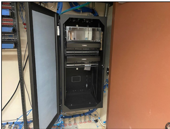
New TR Cabinet
