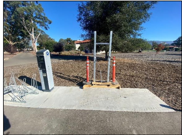
Powered Sign Location
