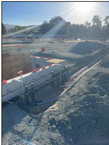
Under Slab Electrical Conduit
