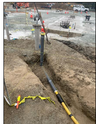
Site Gas Main Line
