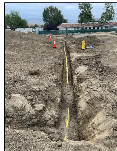
Site Gas Main Line
