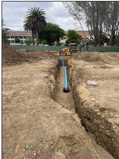
Fire Water Infrastructure
