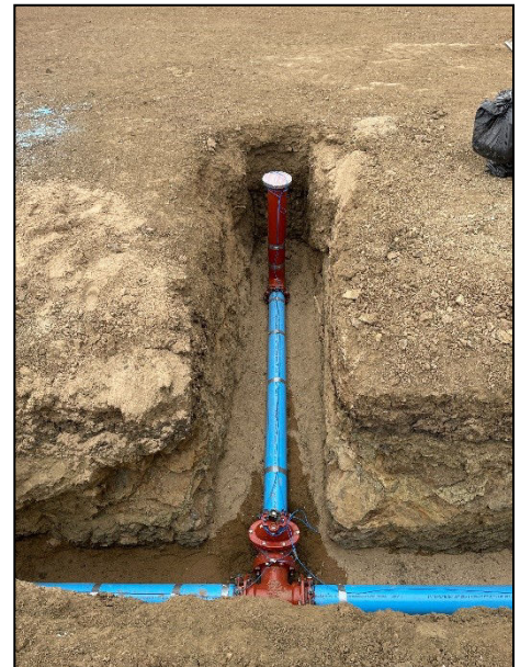
Domestic Water Infrastructure
