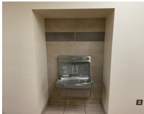
Building 6200 Drinking Fountain
