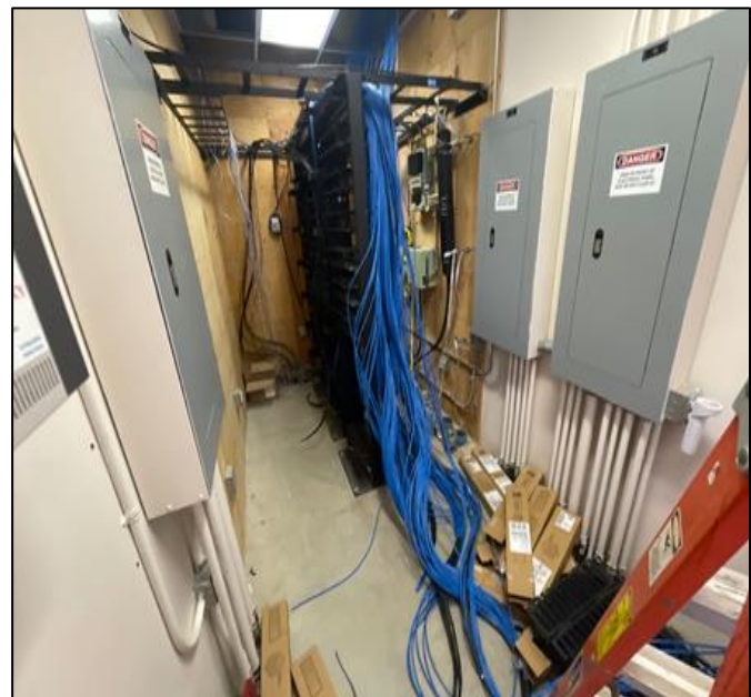
New homeruns to server room
