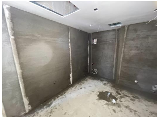
Mortar at Bldg. 6200 restrooms
