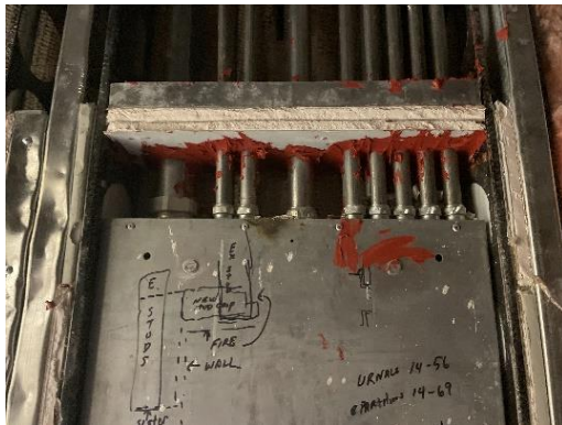
Fire caulking at fire walls
