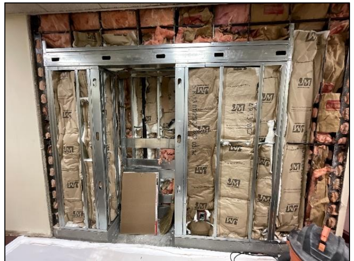
Insulation at drinking fountain alcove
