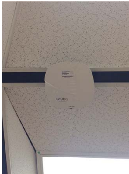
Installed Wireless Access Points
