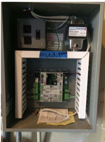
New Control Panels installed in Building 1000 & 1300
