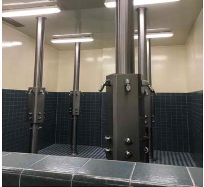
Building 1000 Showers & Freshly Painted Walls
