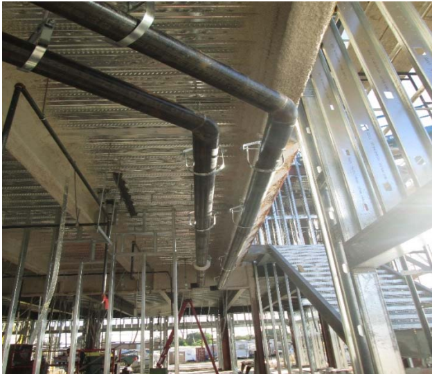
Welded Chilled Water Lines
