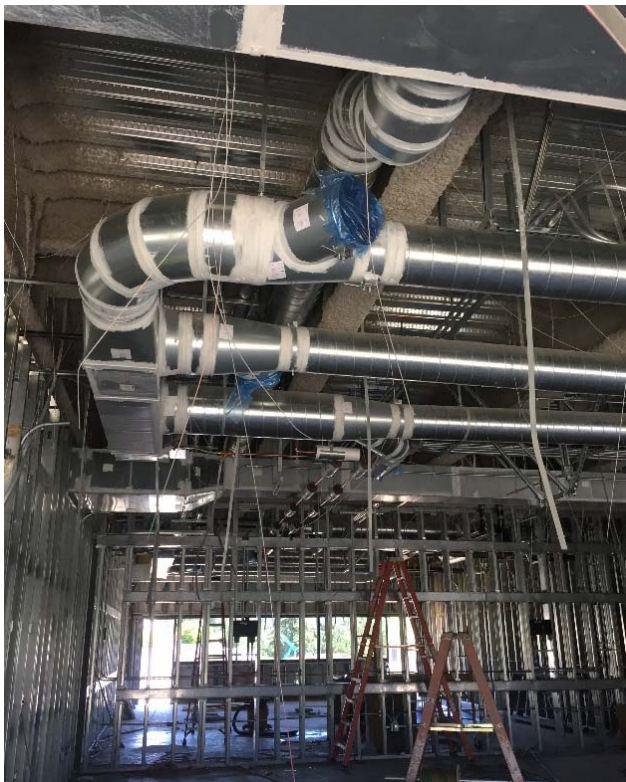
HVAC Equipment in the First Floor Ceiling
