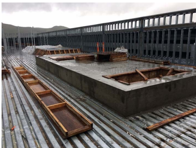
AC Unit Concrete Pads and Curbs on the Roof
