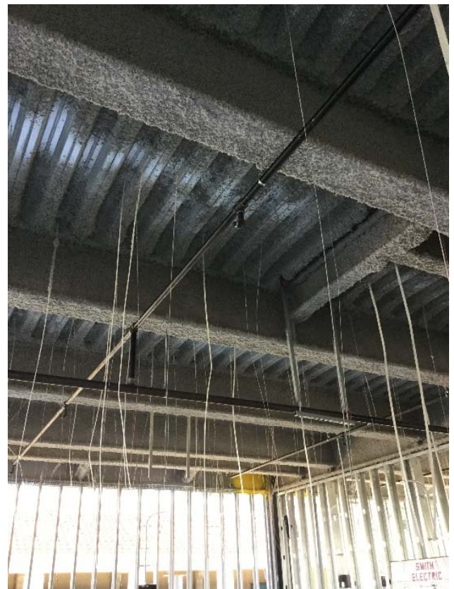
First Floor Fire Sprinkler Piping Rough-In
