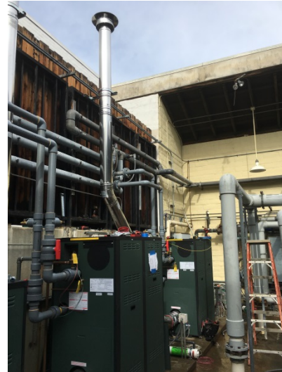
New Boiler Installation
