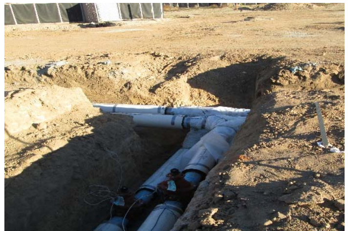
Chilled Water Piping
